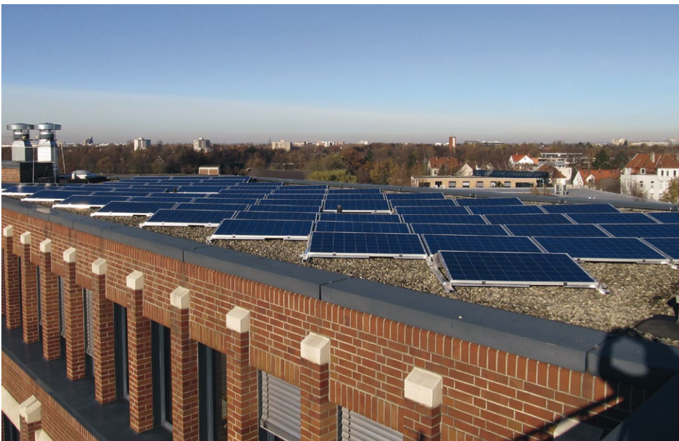
135 kilowatt-peak photovoltaic system on the roof of the main office building at Karl-Wiechert-Allee 50
